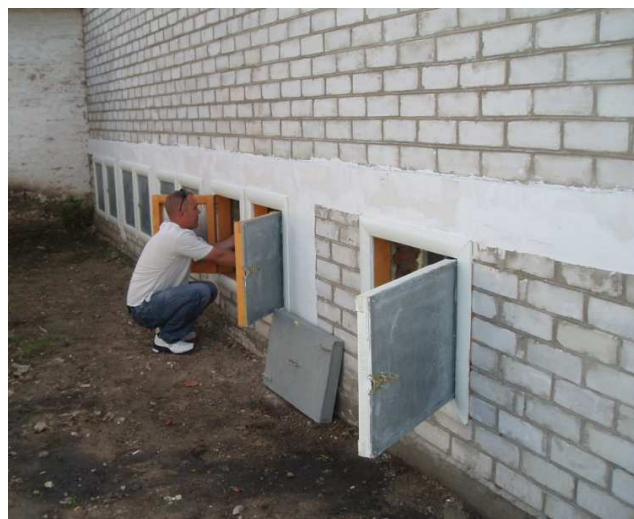
Figure 8: Inspection of the faecal chambers of a UDDT school toilet block in Nizhyn, Ukraine, constructed by the local NGO Mama86 (source: WECF, C. Wendland, 2010).
